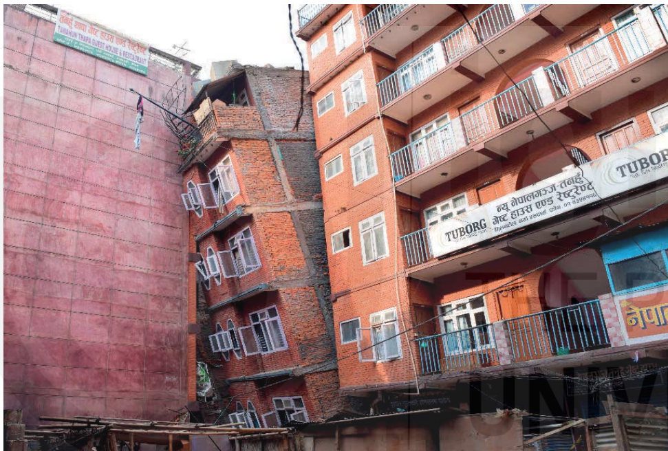
Fig. 6.8: Damage of Buildings by the Earthquake in Kathmandu Valley.
