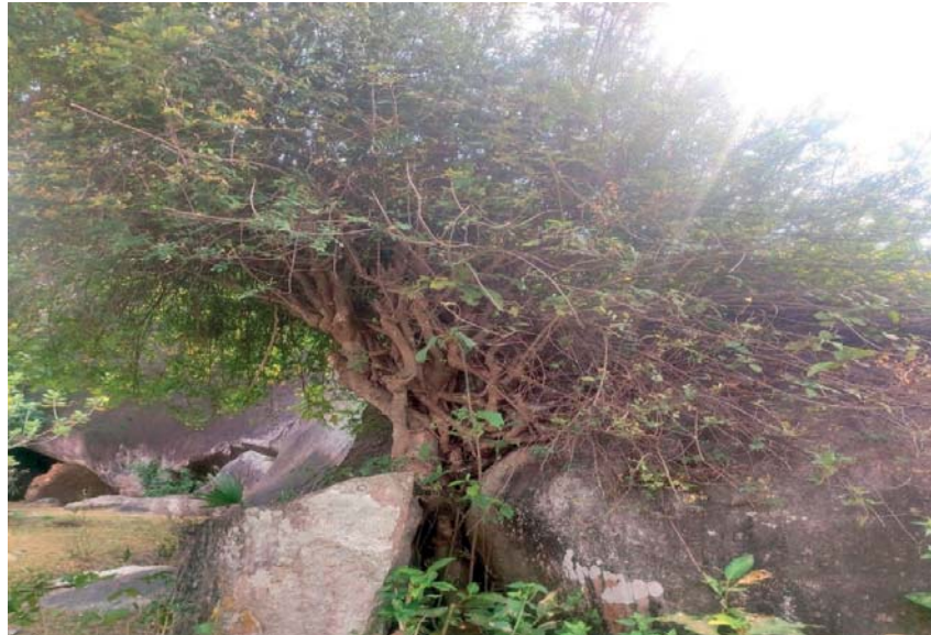
Fig. 7.16: Fractures get widened due to the pressure exerted by the plant causing root wedging leading to the disintegration of the rocks.
