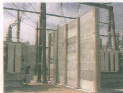
Fig. 2: firewall in electric substation
