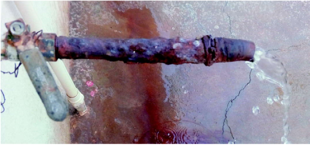
Fig. 8.4: Process of rusting on iron tap.
